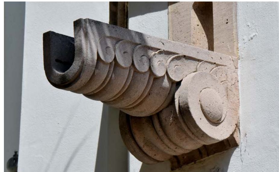
Functional features like this overflow can be detailed in a way to provide architectural interest.
