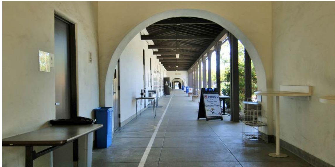
The Schott Center features exposed timber and arched openings to add visual interest to long pedestrian scale arcades – a common Spanish Colonial Revival characteristic.
